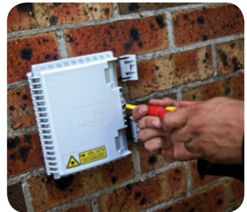
A typical Premises Connection Device, Kiama, New South Wales, one of the First Release Sites.
