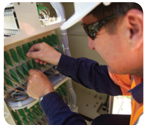
Inside a Fibre Distribution Hub in Kiama, New South Wales, one of the First Release Sites.
