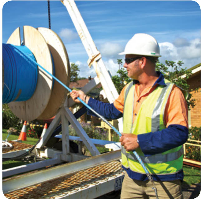
NBN Co or an NBN Co subcontractor will install fibre infrastructure to each premises in a new estate.
