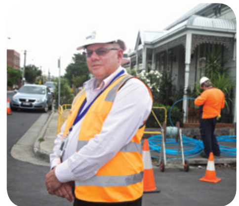
A construction manager in Brunswick, Victoria, one of the First Release Sites.
