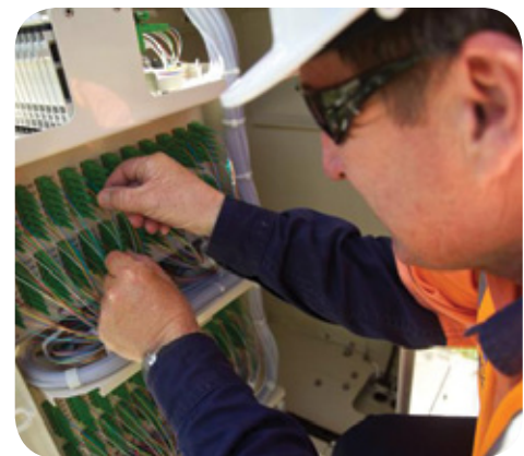
Inside a Fibre Distribution Hub in Kiama, New South Wales.
