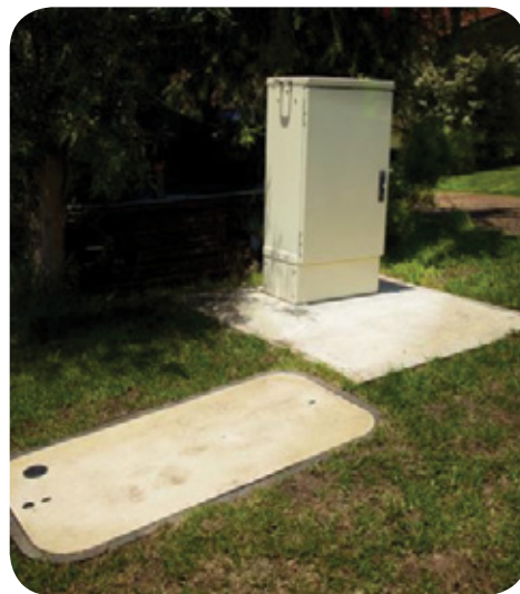
Fibre Distribution Hub and closed pit in Kiama, New South Wales.
